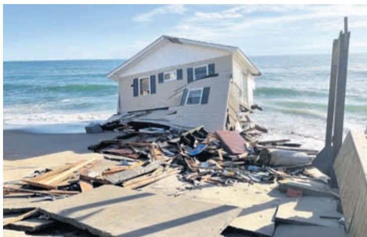
This image released by the National Park Service, shows a collapsed beachfront home along Ocean Drive in Rodanthe, N.C., on Wednesday, Feb. 9, 2022.
